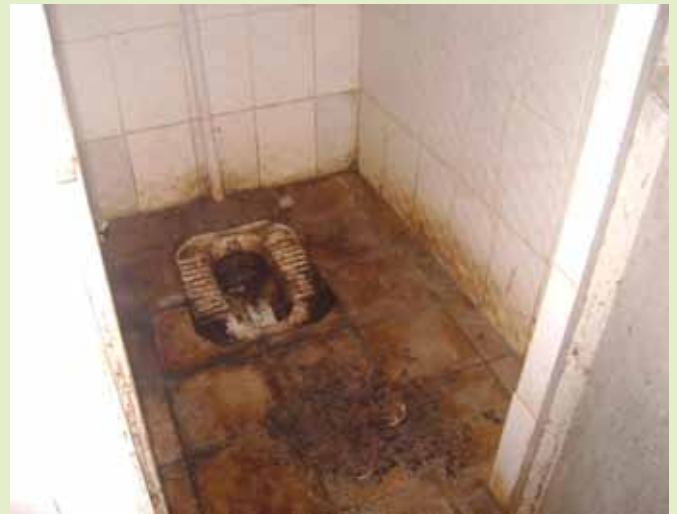
Poor maintenance and cleanliness can lead to girls not using latrines
