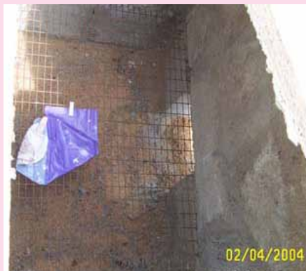
Fire grill inside incinerator
