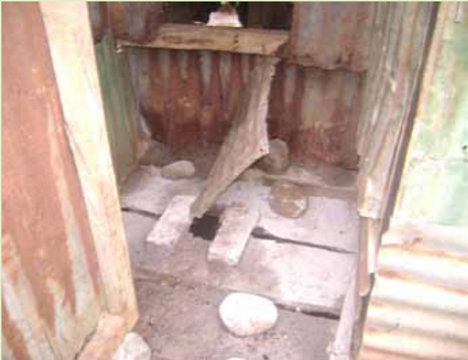
Poor quality latrine with rusty corrugated sheet walling, posing a health and safety hazard
