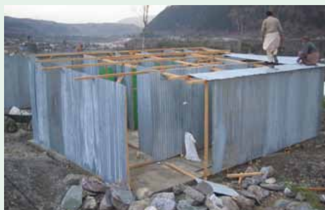
Warm bathing unit under construction – laundry area seen to the front and right of the picture
